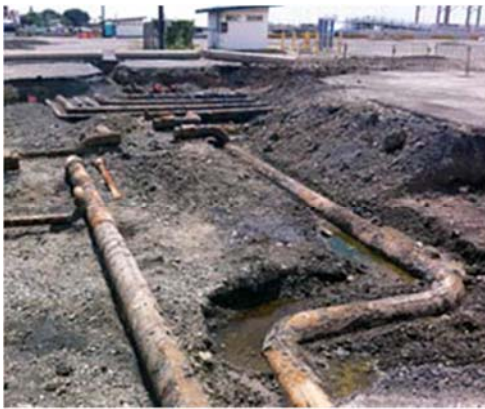
Exposed abandoned pipelines in the harbor area
